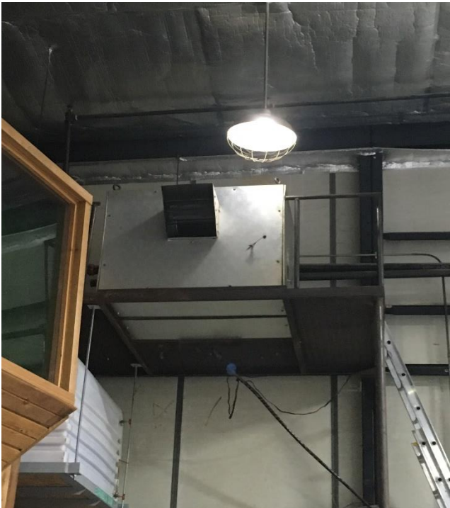
Current Arena Dehumidifier
